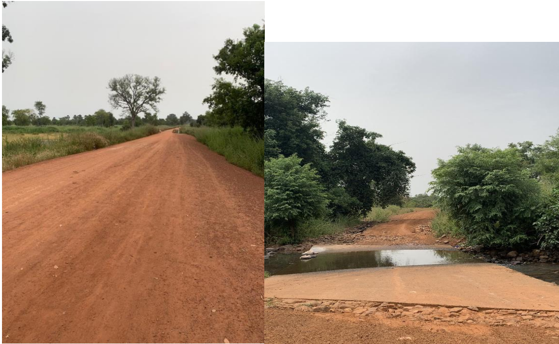
Photo 1: Image of isolated areas with stagnant water and impassable roads in the rainy season
